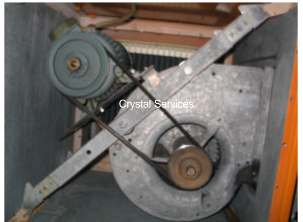
Abluftventilator Pizzeria nachher
